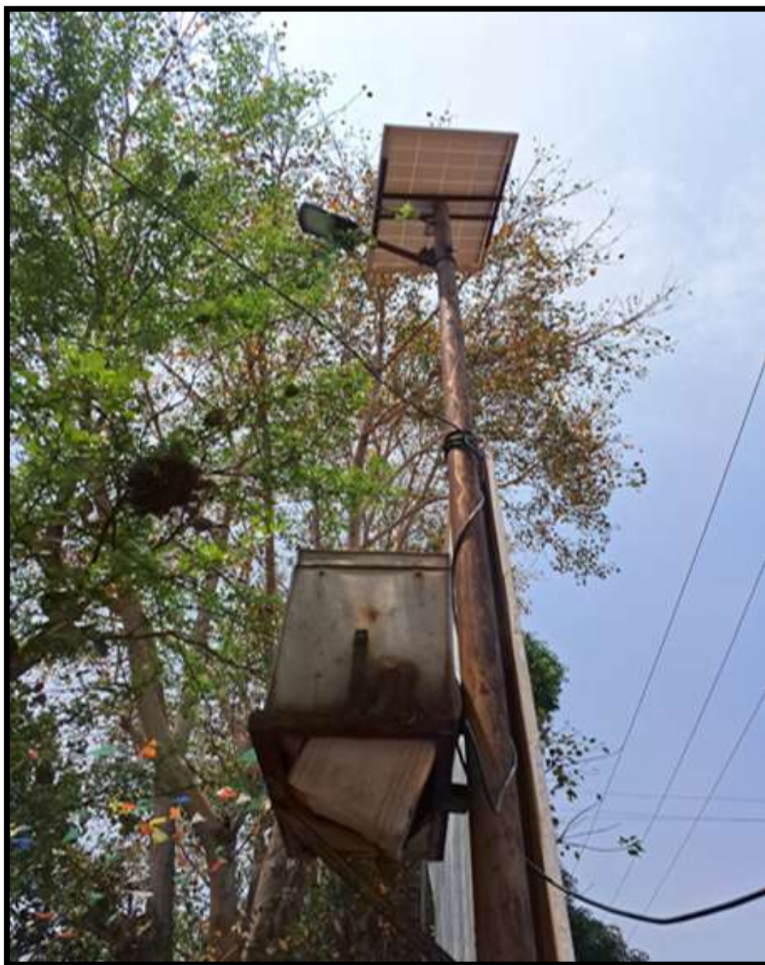
Solar panel fitted in college campus, to generate solar energy for lightening the lts.
